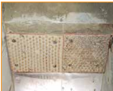
Discharge Chute Primary Crushing
